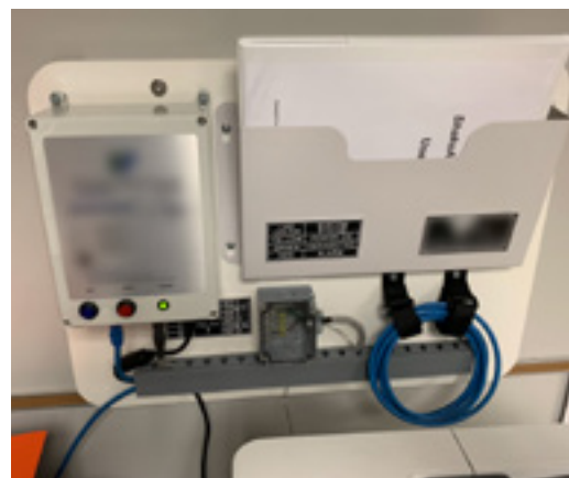
A ShakeAlert-powered box (12 in. by 16 in.) is mounted on the wall in the main office of Stanwood Elementary School in WA. The Stanwood-Camano School District has integrated ShakeAlert EEW into its public address system, so all buildings across its campus are alerted simultaneously. Image is courtesy of Varius, Inc., a ShakeAlert Licensed Operator
