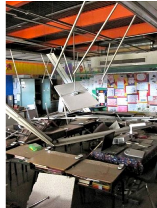
Classroom in Calexico, CA April 2010 M7.2
