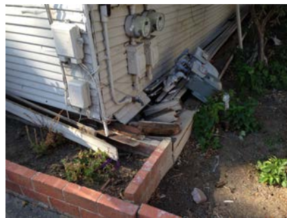
Toppled “cripple wall”
