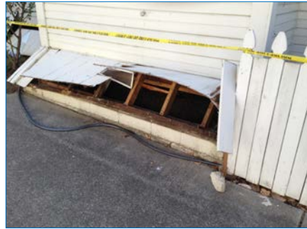
Toppled “cripple wall”
