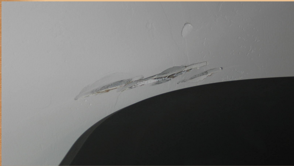
Piano Left Marks on Wall- Lifted up 4-5 Inches
