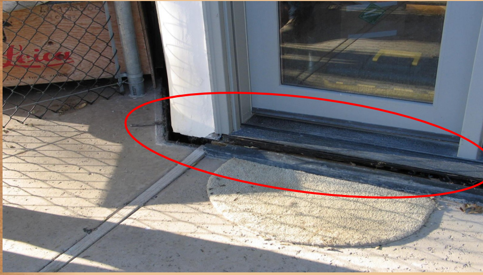
Patio Pulled Away and Dropped About 4”
