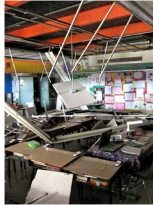
Classroom in Calexico, CA April 2010 M7.2
